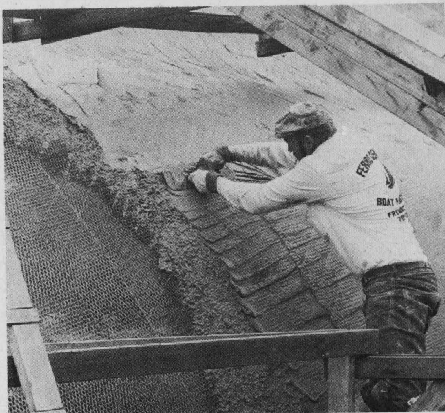
Push, push, push is the action necessary to achieve proper mortar penetration, a prime ingredient for a strong hull. Note the distinct "shingle" pattern caused by the trowel action. Do not attempt to cover the mesh completely at this stage.
