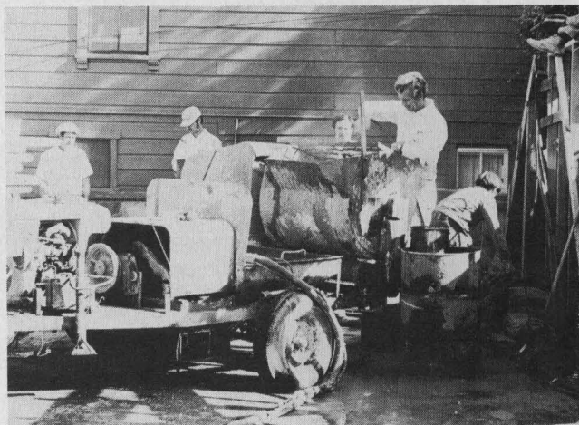
Shortly after sunrise while it is still cool and still, John and his crew prepare the first batch of mud for Flicka.
