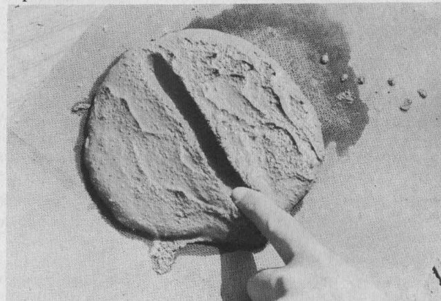
Careful addition of premeasured water will ensure a strong but workable mortar. Note that the mortar leaves a distinct finger impression without filling in. It's a good mix.
