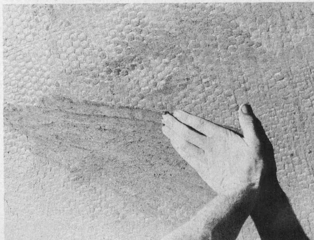
The "palm" test is a good way to determine the right time to apply the skim coat. Allow enough lead time to mix your mortar. This builder has chosen chicken wire mesh at the cost of strength, but his penetration looks perfect.
